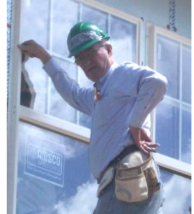
Roger Diggle on the roof, working on the windows (in the photo to the left as well)
